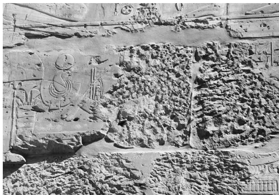
Figure 3. Quarry damage; detail of plate 178
